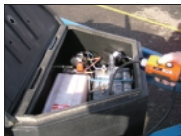
Plastic compartment holds controls, hydraulic pump and battery.*
